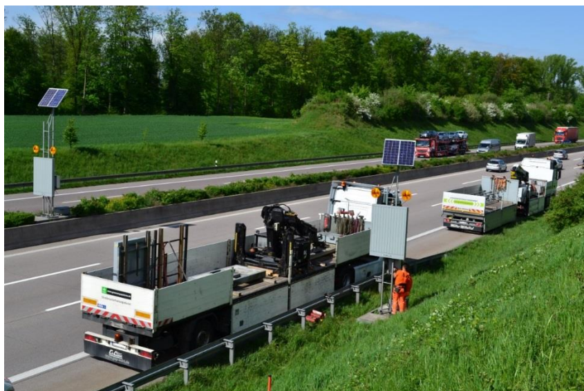
Picture: Installation of the mobile traffic jam warning system on motorway A5 around Baden-Baden (Source: Green Way Systems)
