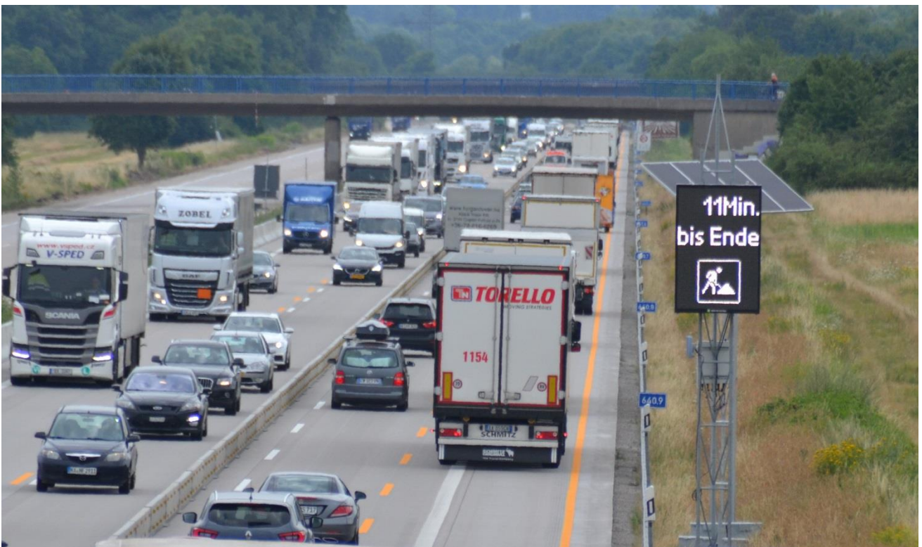
Picture 1: display location in the construction site on motorway A5 (Source: Green Way Systems)
