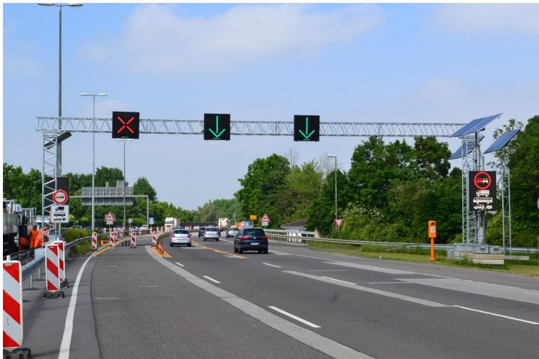
Picture 2: mobile sign gantry with LED lane control signs (source: Green Way Systems)
